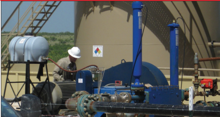
FIELD SERVICE START-UP
